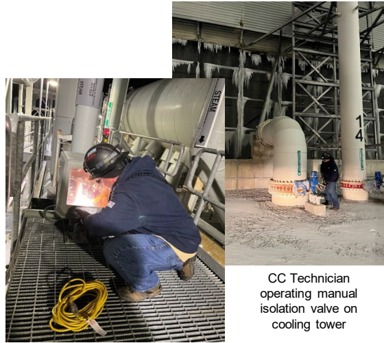
CC Technician adding additional heat to an instrumentation enclosure
