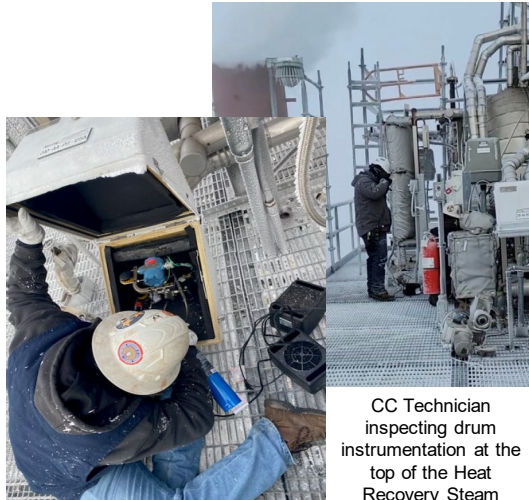
CC Technician thawing a sensing line on a control device
